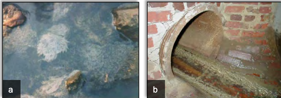
Figure 2 - Sewage. A strong organic or sewage-like odor can indicate a sanitary sewer leak or overflow. Indicators of sewage discharge can include (a) sewage fungus and (b) bacteria growth in outfall.
